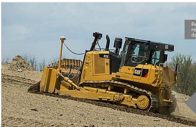
Physical asset operational in the field
